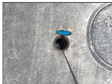
宅地内止水栓 (0.12 \text{m}^3/\text{h} ) No.215 筒内に水
